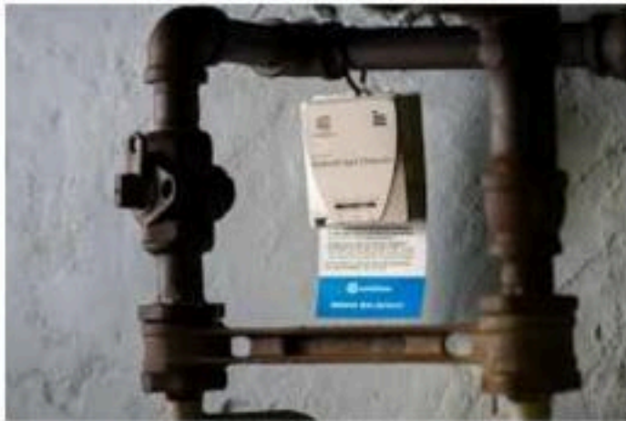
Detectors installed where service enters building
